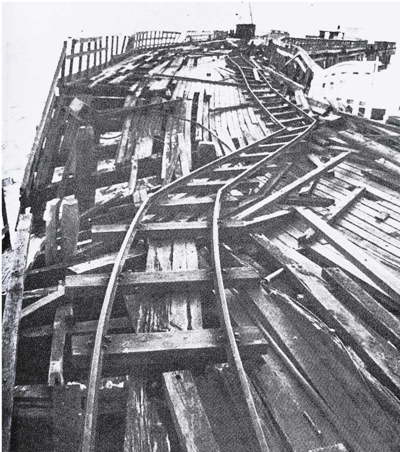
The damage to the Pier and railway following the storm during the night of 11th/12th January 1978. The track has been thrown to the other side of the Pier and badly damaged. The Pier was repaired, but sadly the railway never reopened. ( East Essex Gazette. 13/01/78 )
